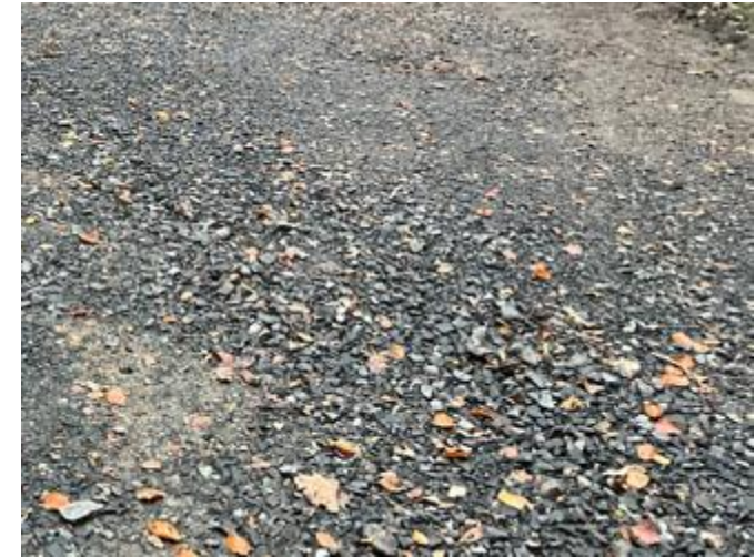
Example of an area of loose grey stones on firm earth creates uneven ground
